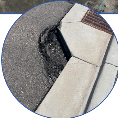
5. Deterioration of Site or Other Improvements
