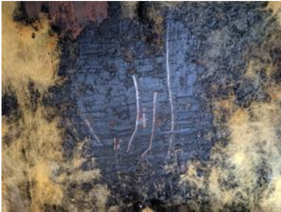
CHE-FTSX812-140721-013 thru 015, 0.42% Asbestos, Black coating
