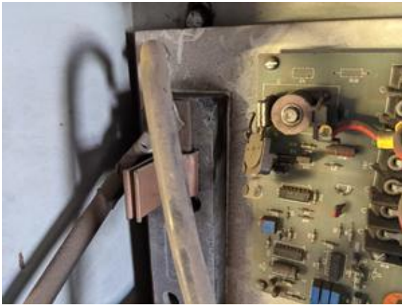
CHE-CNW11097-140721-001 thru 003, 6% Asbestos, Black bakelite
