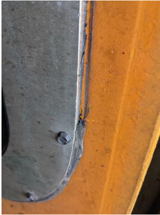
CHE-DRGW01489-150721-001 thru 003, 8% Asbestos, Black window caulk
