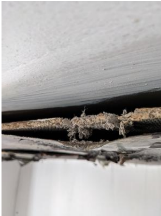
CHE-FTSX812-140721-004 thru 006, 15% Asbestos, Gray transite
