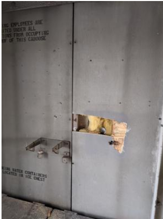
CHE-MP13835-130721-004 thru 006, 10% Asbestos, White coating
