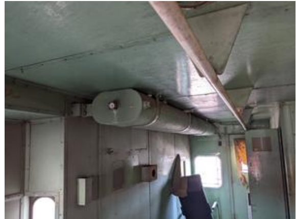
CHE-SP4641-130721-004 thru 006, 10% Asbestos, White/Green Coating
