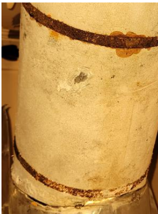
CHE-SP7077-170821-043 thru 045, 30% Asbestos, White exhaust pipe wrap
