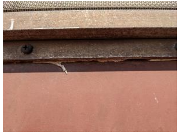
CHE-SP4641-130721-002P, PCB Not Detected, White window caulk
