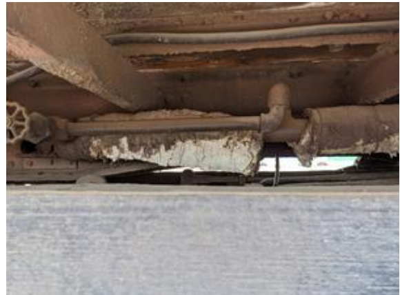
CHE-SP7078-180821-049 thru 051, 15% Asbestos, White pipe wrap
