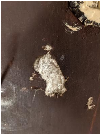
CHE-SP7078-180821-019 thru 021, 65% Asbestos, White fiberboard
