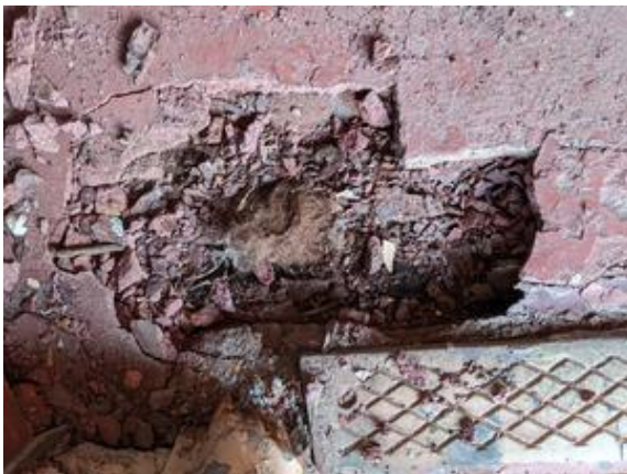
CHE-SP7077-170821-022 thru 024, 0.75% Asbestos, Red cementitious material
