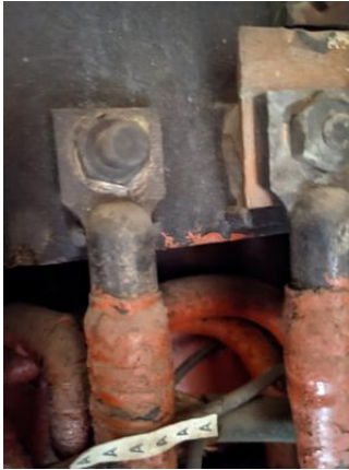
CHE-SP7078-180821-025 thru 027, 6% Asbestos, Black fiberboard
