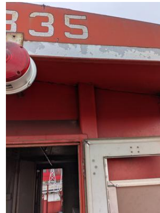
CHE-MP13835-130721-022 thru 024, 10% Asbestos, Gray roof seam sealant
