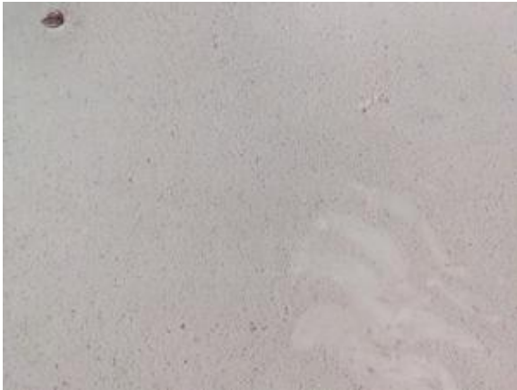
CHE-SP4641-130721-013 thru 015, 10% Asbestos, White wall coating
