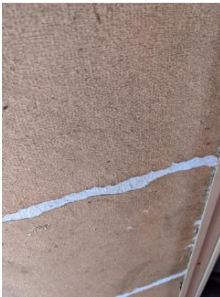
CHE-SP7077-170821-040 thru 042, 65% Asbestos, White Insulation
