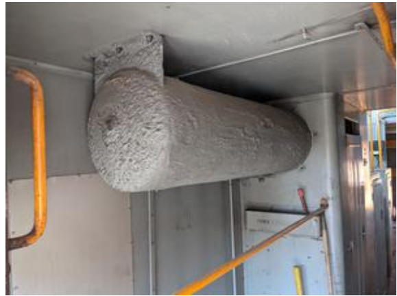
CHE-DRGW01524-170721-010 thru 012, 6.42% Asbestos, White coating
