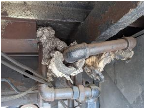
CHE-SP7078-180821-049 thru 051, 15% Asbestos, White pipe wrap
