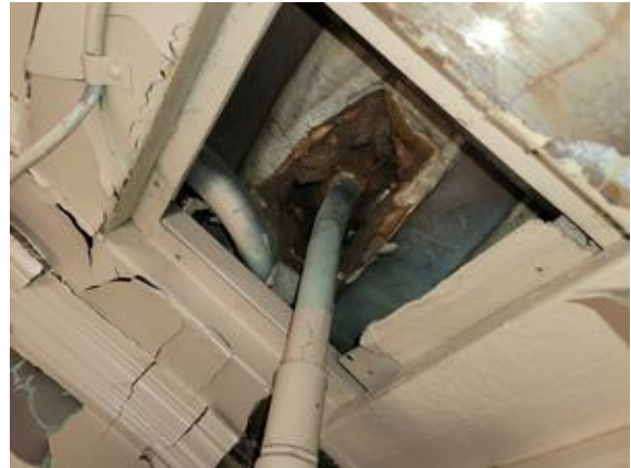
CHE-SP7077-170821-010 thru 012, 40% Asbestos, Gray Insulation
