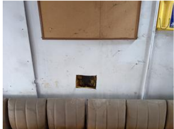
CHE-FTSX812-140721-013 thru 015, 0.42% Asbestos, Black coating
