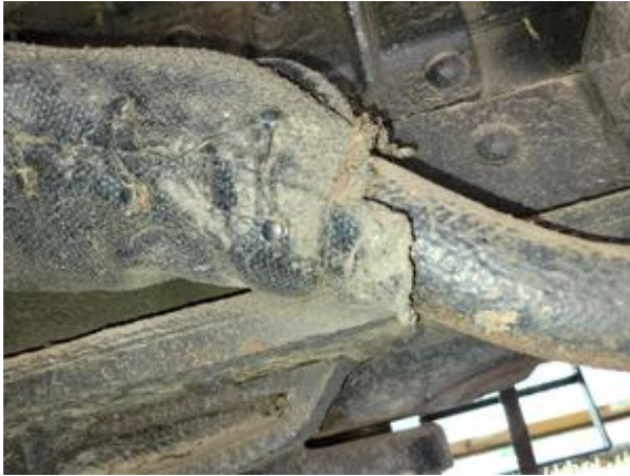
CHE-SP7077-170821-016 thru 018, 30% Asbestos, White pipe wrap
