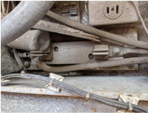
CHE-CNW11111-150721-001 thru 003, 6% Asbestos, Black bakelite
