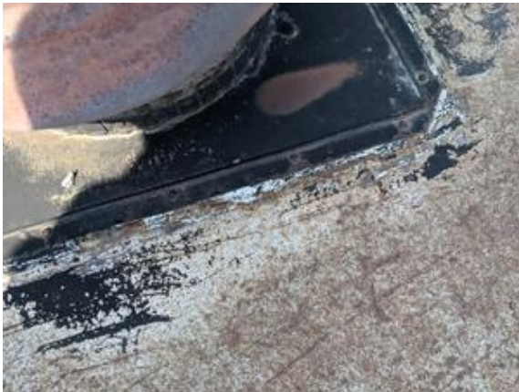
CHE-DRGW01481-160721-007 thru 009, 2.85% Asbestos, White/brown sealant
