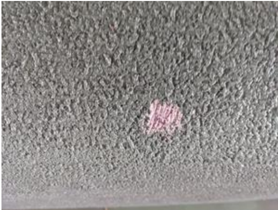
CHE-SP4641-130721-004 thru 006, 10% Asbestos, White/Green Coating
