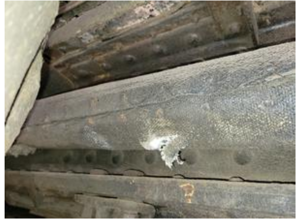
CHE-SP7077-170821-016 thru 018, 30% Asbestos, White pipe wrap
