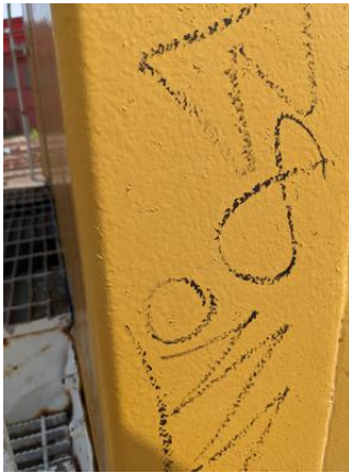
CHE-CNW11047-150721-002L, 0.45% Lead, Yellow
