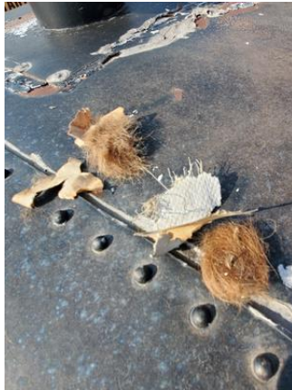
CHE-SP7077-170821-010 thru 012, 40% Asbestos, Gray Insulation
