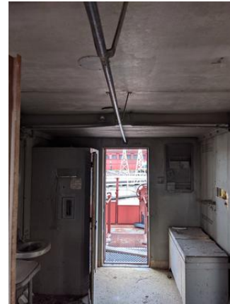
CHE-MP13835-130721-013 thru 015, 10% Asbestos, White coating
