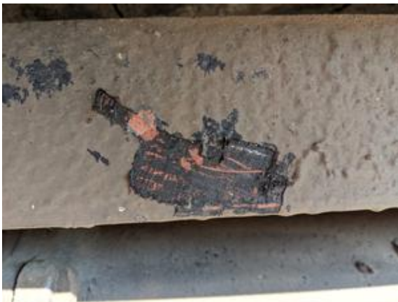
CHE-RI17017-150721-004 thru 006, 15% Asbestos, Black fire proofing
