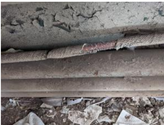
CHE-SP7078-180821-040 thru 042, 55% Asbestos, Beige pipe wrap
