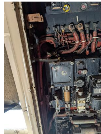
CHE-SP7078-180821-031 thru 033, Asbestos Not Detected, Gasket (layered silver coating and black felt)
