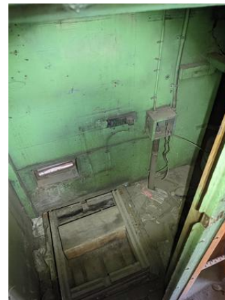
CHE-DRGW01489-150721-007 thru 009, Asbestos Not Detected, Breakers
