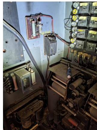
CHE-SP7077-170821-034 thru 036, 1.59% Asbestos, Black bakelite
