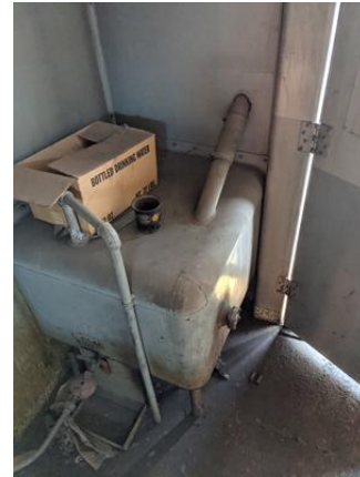
CHE-DRGW01524-170721-013 thru 015, 1.43% Asbestos, Tan sealant
