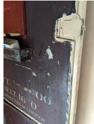
CHE-SP7078-180821-019 thru 021, 65% Asbestos, White fiberboard
