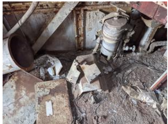
CHE-UP928-160821-025 thru 027, 20% Asbestos, Gray transite
