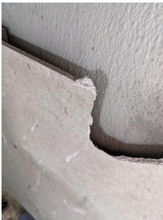
CHE-MP13835-130721-016 thru 018, 15% Asbestos, Gray transite boards
