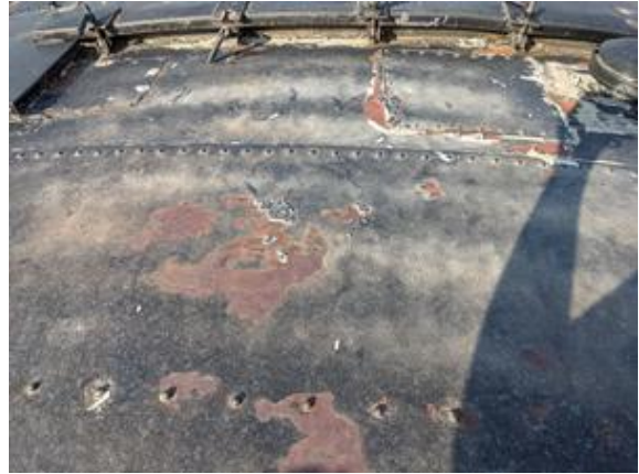
CHE-SP7077-170821-001 thru 003, 6% Asbestos, Silver/black coating
