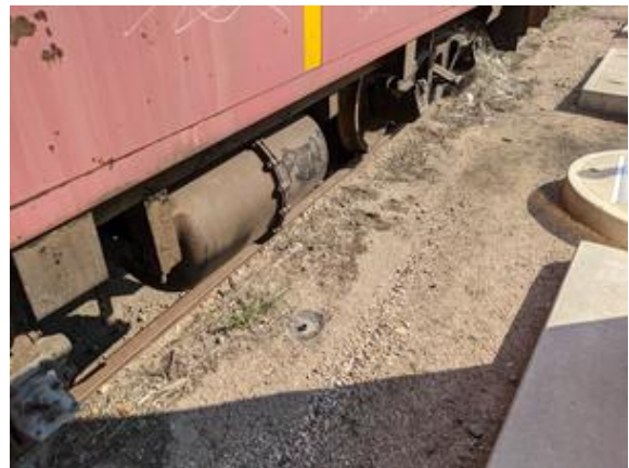
CHE-RI17017-150721-004 thru 006, 15% Asbestos, Black fire proofing
