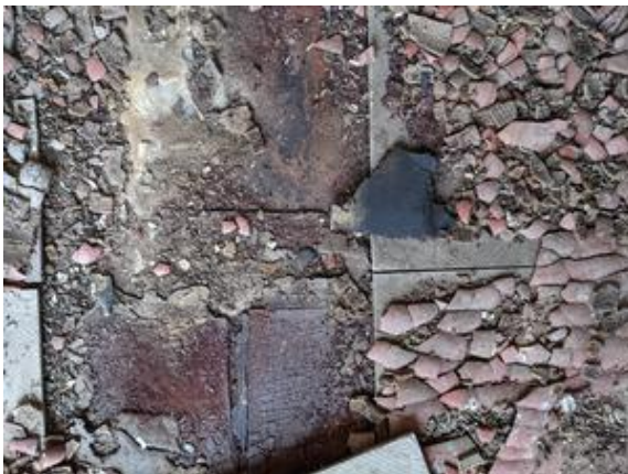
CHE-SP7078-180821-013 thru 015, Asbestos Not Detected, Yellow mastic associated with gray 9"x9" floor tile
