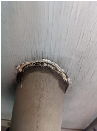
CHE-DRGW01524-170721-013 thru 015, 1.43% Asbestos, Tan sealant
