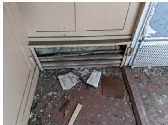
CHE-SP7078-180821-040 thru 042, 55% Asbestos, Beige pipe wrap
