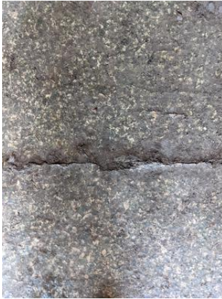
CHE-DRGW01524-170721-001 thru 003, Asbestos Not Detected, Beige flooring and gray mastic
