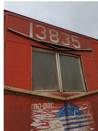
CHE-MP13835-130721-001P, PCB Not Detected, Gray window caulk
