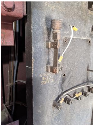
CHE-UP928-160821-007 thru 009, 40% Asbestos, Black Fireboard
