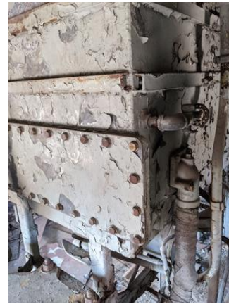
CHE-UP928-160821-010 thru 012, Asbestos Not Detected, Gray/Brown Gaskets
