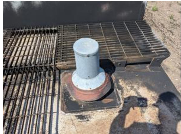
CHE-DRGW01481-160721-007 thru 009, 2.85% Asbestos, White/brown sealant
