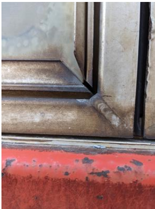
CHE-MP13835-130721-001P, PCB Not Detected, Gray window caulk
