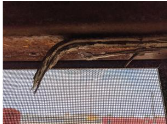
CHE-SP4641-130721-001P, PCB Not Detected, White window caulk
