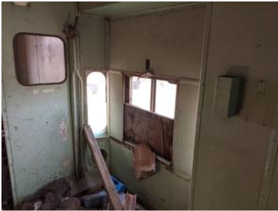
CHE-SP4641-130721-001P, PCB Not Detected, White window caulk
