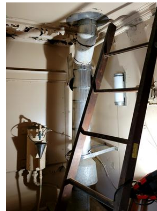
CHE-SP7077-170821-043 thru 045, 30% Asbestos, White exhaust pipe wrap
