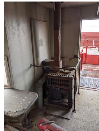
CHE-MP13835-130721-016 thru 018, 15% Asbestos, Gray transite boards
