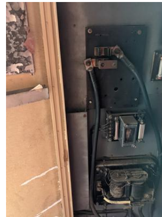
CHE-SP7077-170821-040 thru 042, 65% Asbestos, White Insulation
