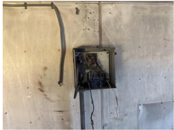
CHE-CNW11097-140721-001 thru 003, 6% Asbestos, Black bakelite
