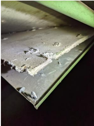
CHE-DRGW01489-150721-004 thru 006, 60% Asbestos, White fiberboard
