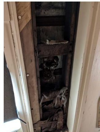
CHE-SP7078-180821-007 thru 009, 15% Asbestos, White/brown paper insulation
