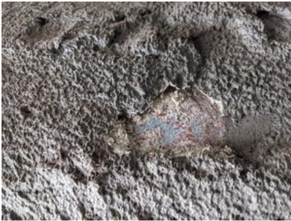
CHE-DRGW01524-170721-010 thru 012, 6.42% Asbestos, White coating
