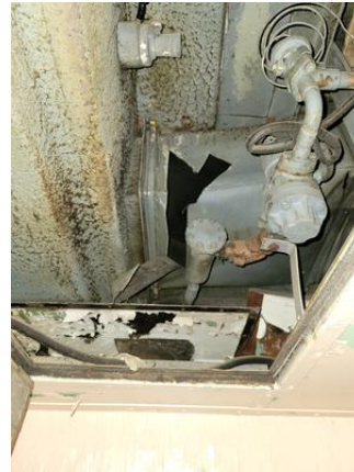
CHE-SP7077-170821-031 thru 033, 6% Asbestos, Black wall coating
