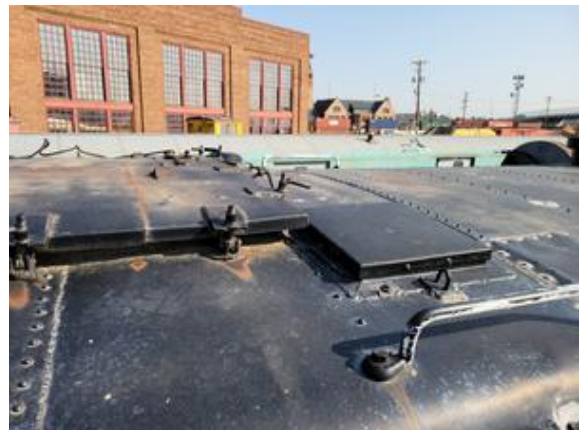
CHE-SP7077-170821-013 thru 015, Asbestos Not Detected, Thin black/gray coating
