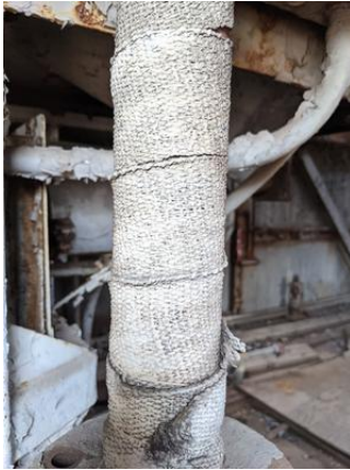
CHE-UP928-160821-001 thru 003, 90% Asbestos, White pipe wrap
