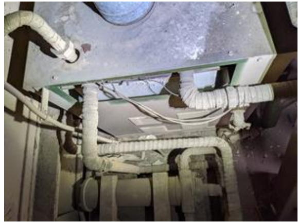
CHE-SP7077-170821-046 thru 048, 10% Asbestos, Gray heater block
