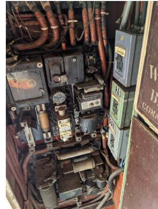
CHE-SP7078-180821-028 thru 030, 15% Asbestos, Black bakelite
