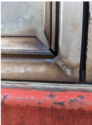
CHE-MP13835-130721-025 thru 027, 10% Asbestos, Gray window caulk
