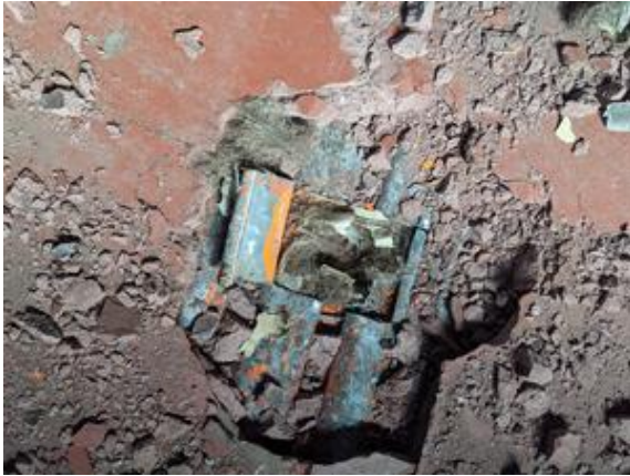
CHE-SP7078-180821-016 thru 018, 1.75% Asbestos, Red cementitious flooring
