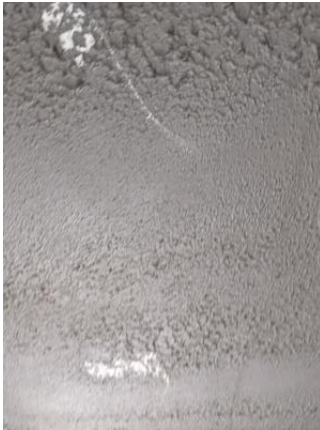
CHE-MP13835-130721-013 thru 015, 10% Asbestos, White coating
