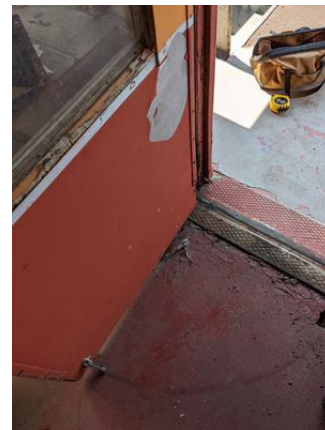
CHE-SP7077-170821-022 thru 024, 0.75% Asbestos, Red cementitious material
