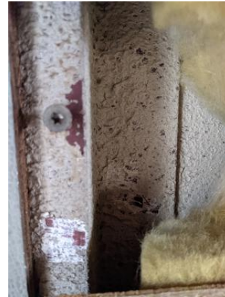
CHE-MP13835-130721-004 thru 006, 10% Asbestos, White coating
