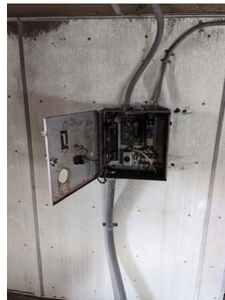
CHE-CNW11047-150721-007 thru 009, 15% Asbestos, Black bakelite
