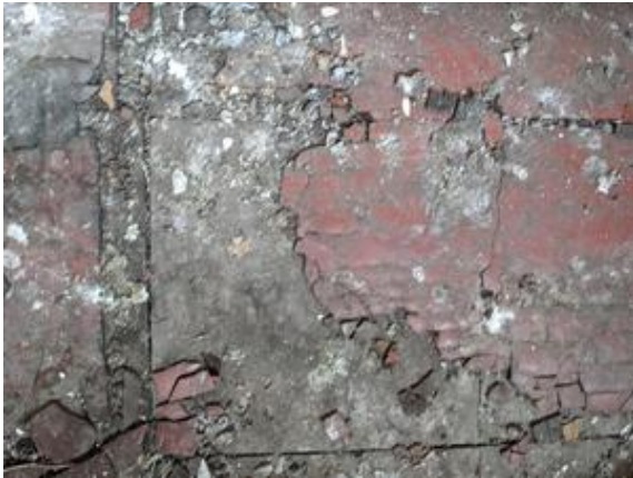
CHE-SP7078-180821-013 thru 015, 6% Asbestos, Gray 9"x9" floor tile and gray leveling compound
