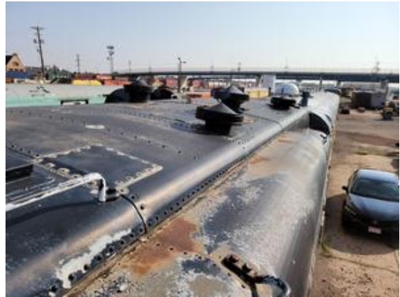
CHE-SP7077-170821-004 thru 005, 8% Asbestos, Black tar
