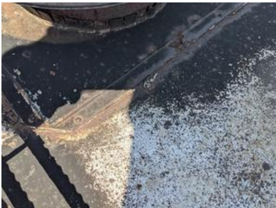
CHE-DRGW01486-160721-007 thru 009, 8% Asbestos, Brown/white sealant
