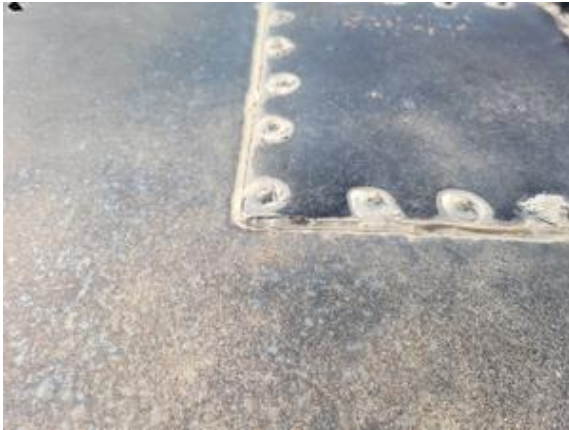
CHE-SP7077-170821-004 thru 005, 8% Asbestos, Black tar
