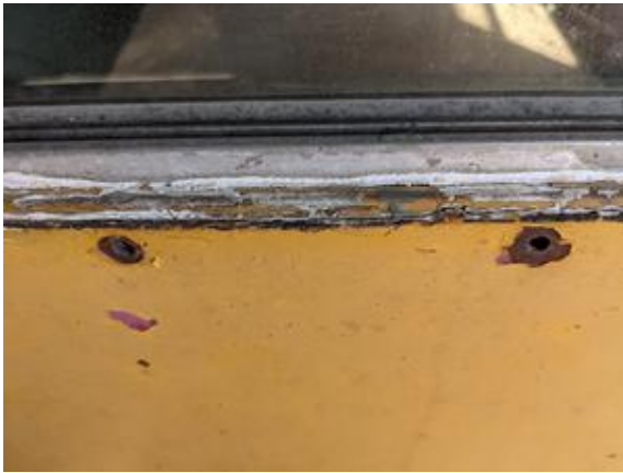
CHE-RI17017-150721-001 thru 003, 1.75% Asbestos, White window glazing
