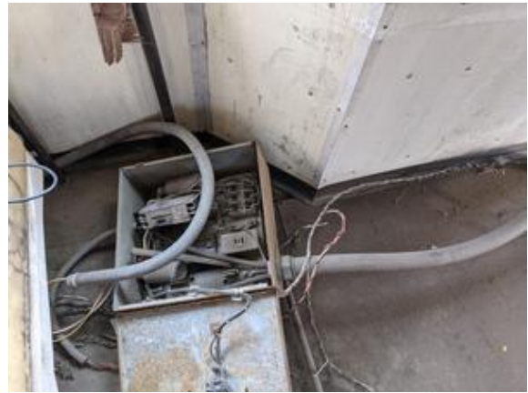
CHE-CNW11111-150721-001 thru 003, 6% Asbestos, Black bakelite
