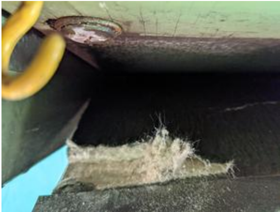
CHE-DRGW01476-170721-004 thru 006, Asbestos Not Detected, Brown fiberboard
