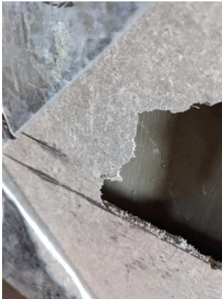
CHE-DRGW01524-170721-004 thru 006, 15% Asbestos, Gray transite boards
