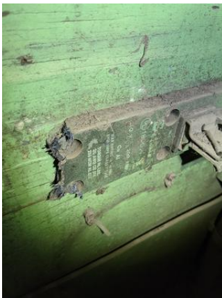
CHE-DRGW01489-150721-007 thru 009, Asbestos Not Detected, Breakers
