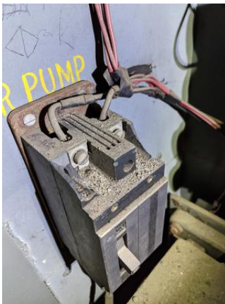
CHE-SP7077-170821-034 thru 036, 1.59% Asbestos, Black bakelite
