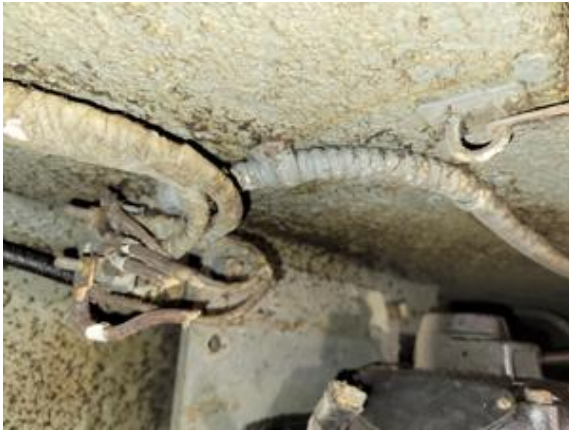
CHE-SP7077-170821-031 thru 033, 6% Asbestos, Black wall coating
