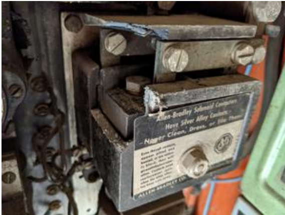
CHE-SP7078-180821-028 thru 030, 15% Asbestos, Black bakelite
