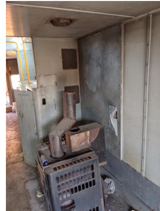
CHE-DRGW01524-170721-004 thru 006, 15% Asbestos, Gray transite boards
