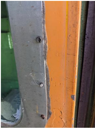
CHE-DRGW01476-170721-001 thru 003, 6% Asbestos, Gray/black window caulk
