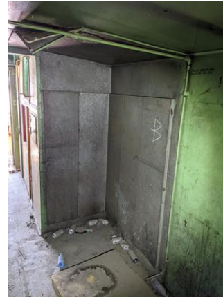
CHE-DRGW01489-150721-004 thru 006, 60% Asbestos, White fiberboard
