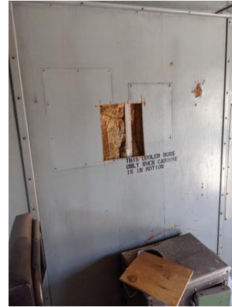
CHE-DRGW01524-170721-019 thru 021, 4.7% Asbestos, White coating
