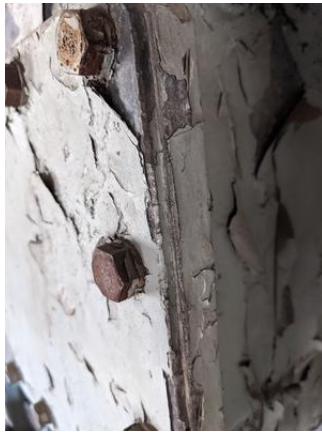
CHE-UP928-160821-010 thru 012, Asbestos Not Detected, Gray/Brown Gaskets
