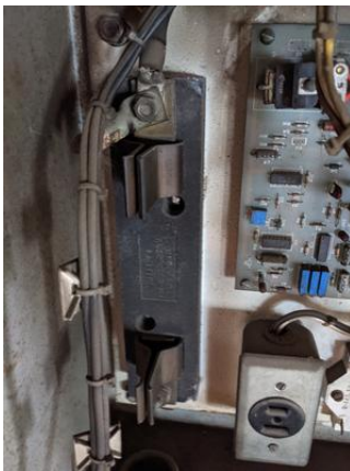
CHE-CNW11047-150721-007 thru 009, 15% Asbestos, Black bakelite
