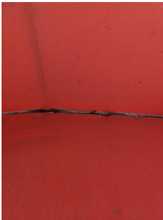
CHE-MP13835-130721-022 thru 024, 10% Asbestos, Gray roof seam sealant
