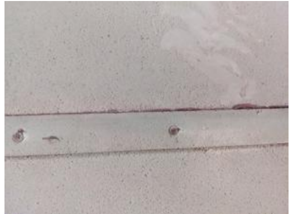
CHE-SP4641-130721-013 thru 015, 10% Asbestos, White wall coating
