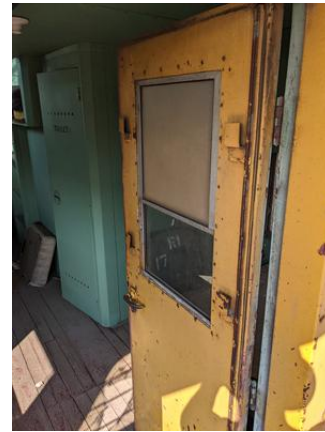
CHE-RI17017-150721-001 thru 003, 1.75% Asbestos, White window glazing
