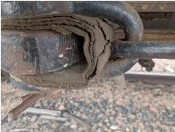
CHE-SP7078-180821-046 thru 048, Asbestos Not Detected, Vibration dampener and mastic
