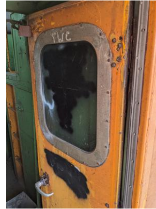
CHE-DRGW01489-150721-001 thru 003, 8% Asbestos, Black window caulk
