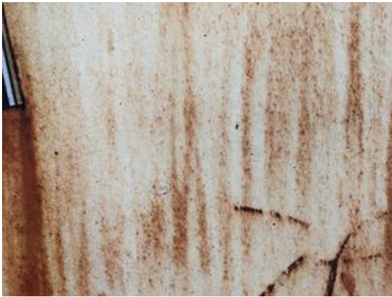
CHE-CNW11111-150721-002L, 5.1% Lead, Yellow
