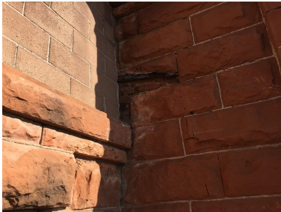
Figure 3 Stone detail at area where Second Floor was added. Note non-historic concrete masonry units. Also note where flashing of the original roofing was let-in at the adjoining stone veneer.
